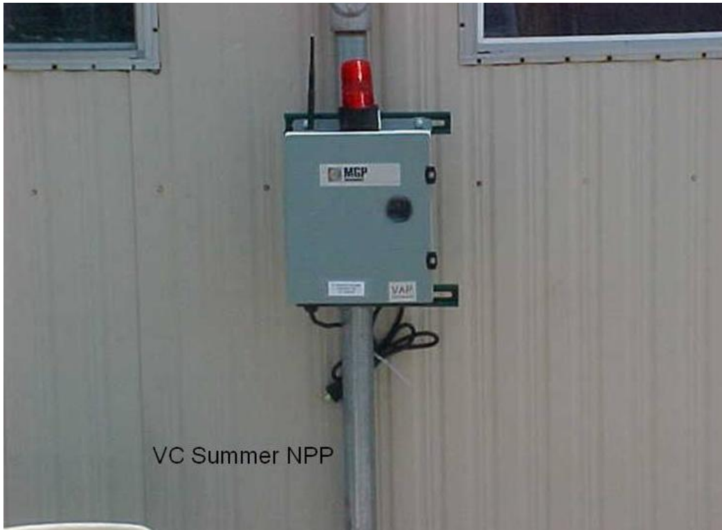
Figure 19 - DRM WRM2-Capable RMD - Auxiliary Building Roof - V.C. Summer NPP (US) 21
